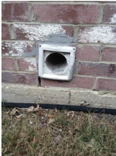
The dryer vent exterior cover is missing
