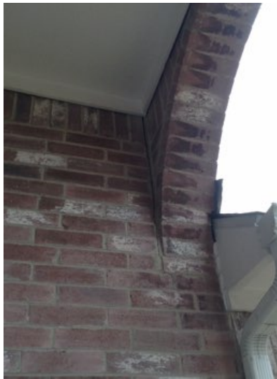
Slightly larger than typical exterior wall cracking was observed. The amount of movement does not suggest a serious structural problem. This area should, of course, be monitored. The rate of movement cannot be predicted during a one-time inspection. Front entry and right corner facing out the front door.
