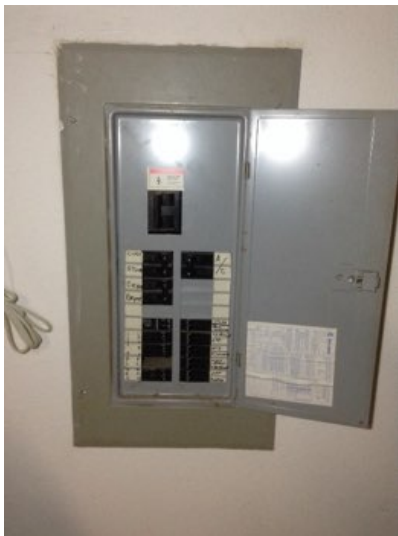
Any openings in the main panel should be covered. Clips can be added to avoid vermin entry points and danger of hands entering the open area.
