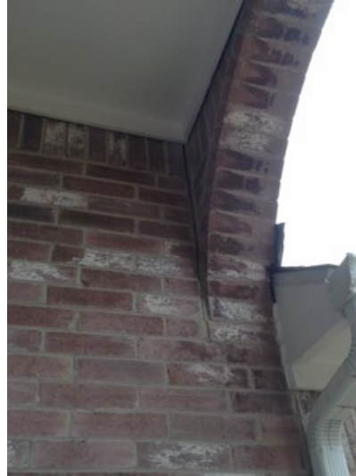
Slightly larger than typical exterior wall cracking was observed. The amount of movement does not suggest a serious structural problem. This area should, of course, be monitored. The rate of movement cannot be predicted during a one-time inspection. Front entry and right corner facing out the front door.
