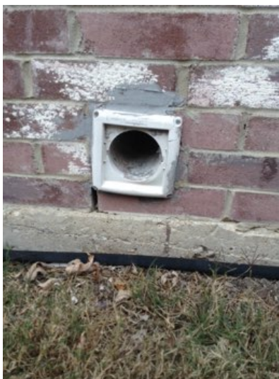
The dryer vent exterior cover is missing
