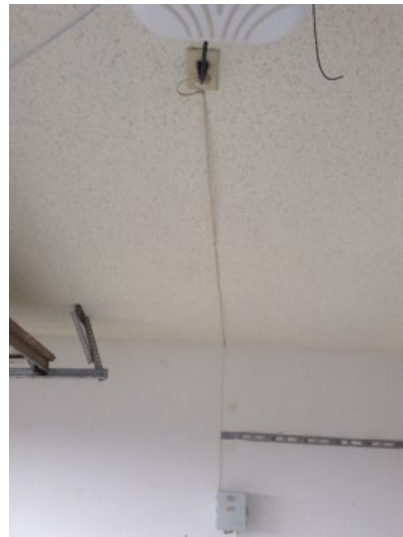
The wiring for the sprinkler system control box is improper and should be repaired. The unit is wired with an extension cord.
