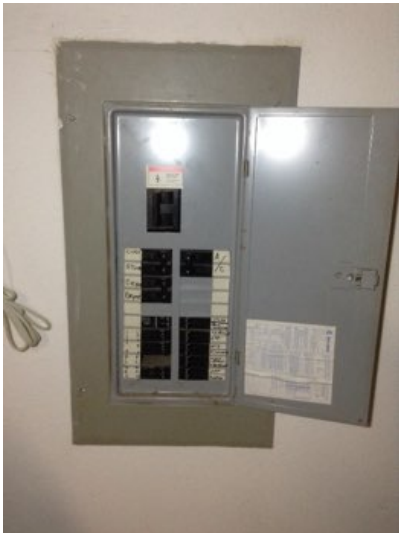
Any openings in the main panel should be covered. Clips can be added to avoid vermin entry points and danger of hands entering the open area.
