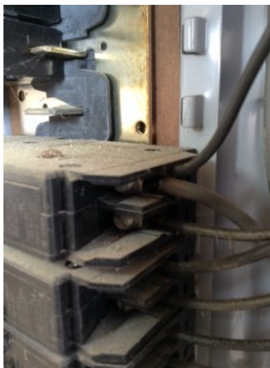
Circuits within the main distribution panel that are doubled up (referred to as "double taps") should be separated. Each circuit should be served by a separate fuse or breaker. This needs to be corrected by a licensed electrician.
